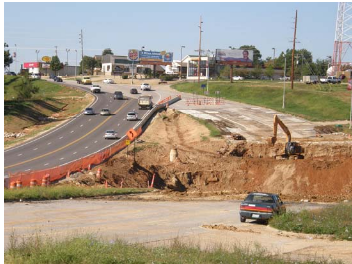
Construction of the Osage Beach Parkway North overpass over the new Rte 54 Expressway.
